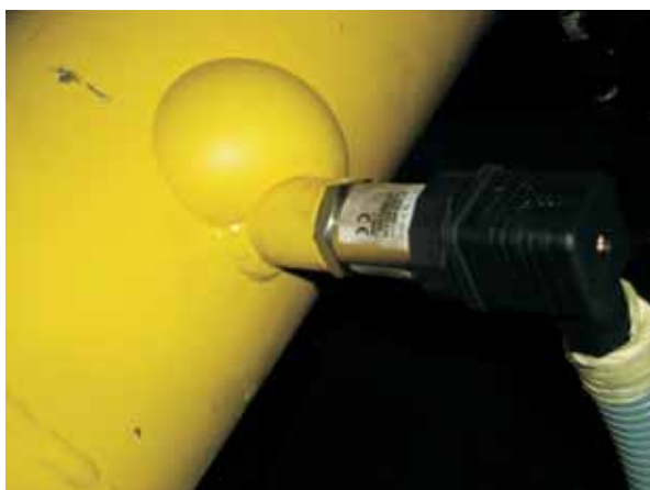
The paint layer temporarily covers the bad weld of the gas line.
