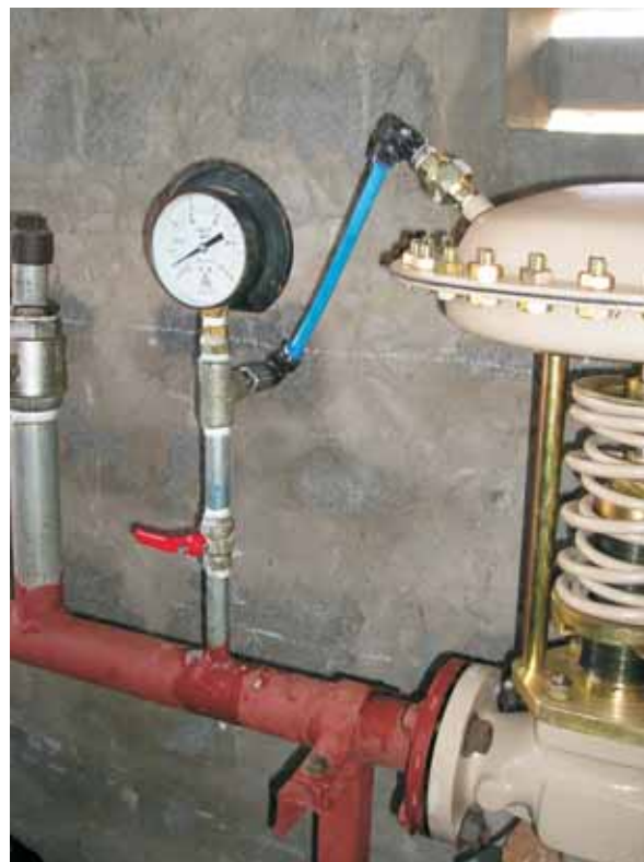
Totally nonsensical shut-off on the gas governor. I persuaded the author for a long time that the shut-off must be still open and not only during reading gas pressure.
